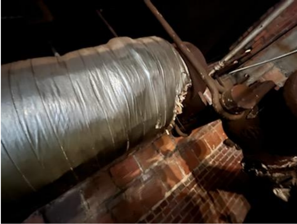
View of ACM Pipe Insulation under Duct Tape
